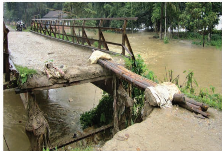
Narayanpur- Old age Bridge broken due to heavy rain
